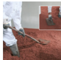
Rework the connecting edges at the wall and compact the applied surface.
